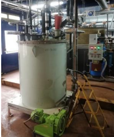
Figure 6. Leaching reactor at the MYTILINEOS pilot plant.
